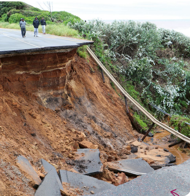
The M4 freeway near Tongaat, Durban, was washed away during the KwaZulu-Natal floods of 21 May 2022, illustrating the severe impact of flooding on critical transport infrastructure.
