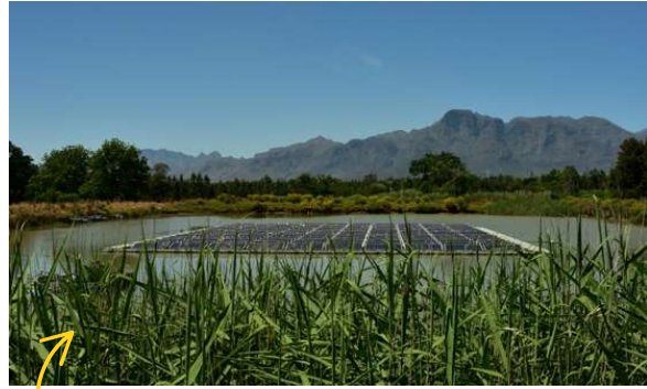
A floating solar station on a farm dam saves arable land and helps against evaporation, Western Cape.
