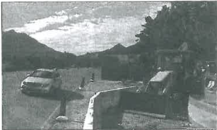
HOTSPOT: The construction site on on Chapmans Peak Drive. PICTURE: DAVID RITCHIE
