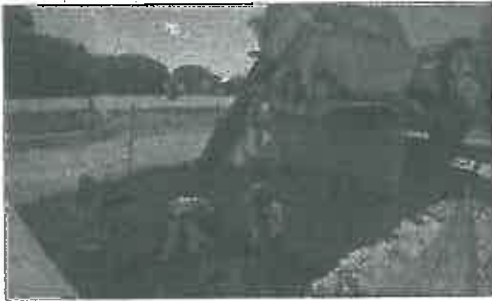
DIGGING IT: Builders hard at work on the Chapman's Peak toll plaza, which is going ahead despite objections from several groups.
